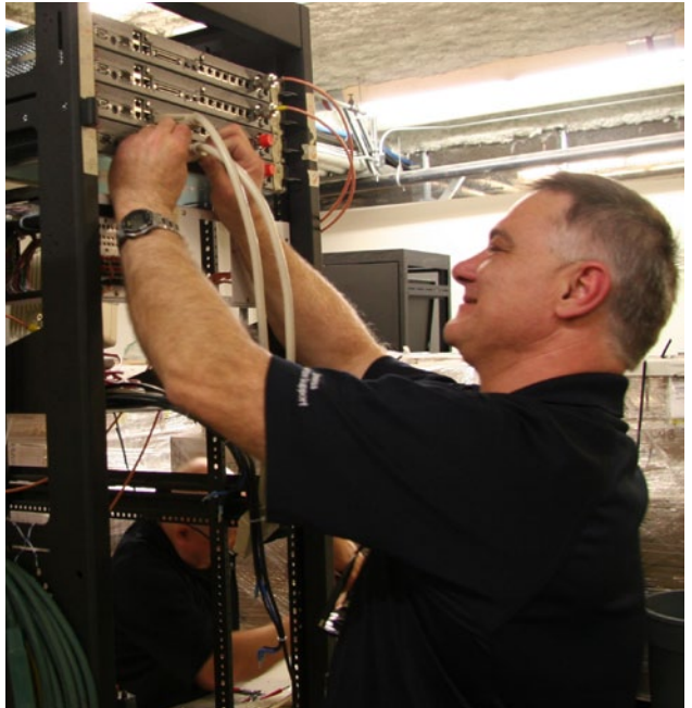
Wireless Technician Trevor Buchholz working on one of the new microwave units at E-Comm, which are significantly smaller than the previous microwave units.
