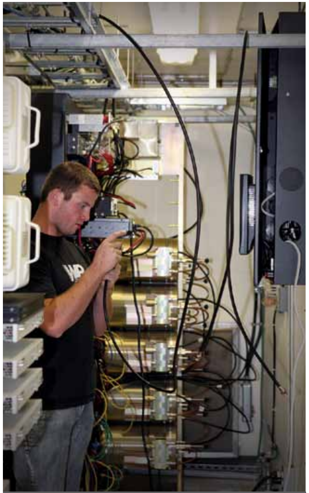
Wireless technician Craig Hayman installs a Locution lead box as part of the new fire-hall alerting system.
